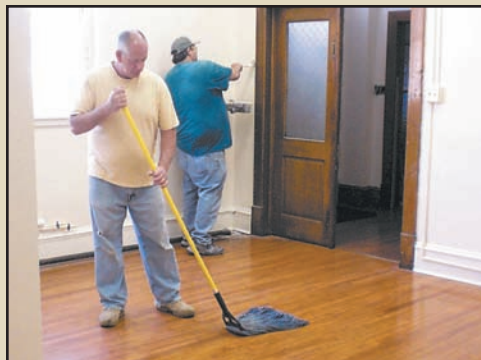
Workman put the finishing touches on the restoration of the church basement auditorium at Sacred Heart Parish, Phoenixville. The parish raised 138% of their goal, providing more funds to address renovation and repair projects in the century-old Church.
